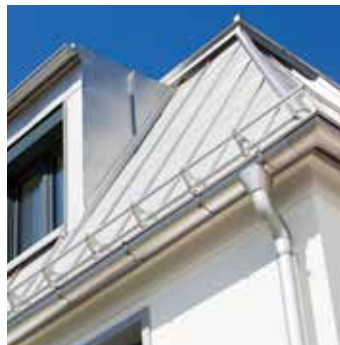
Roof drainage system
