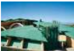
Pilgrimage Church Padre Pio, San Giovanni Rotondo, I Renzo Piano Building Workshop, Genoa WAL S.r.l., Bregnano (CO) TECU® Patina
